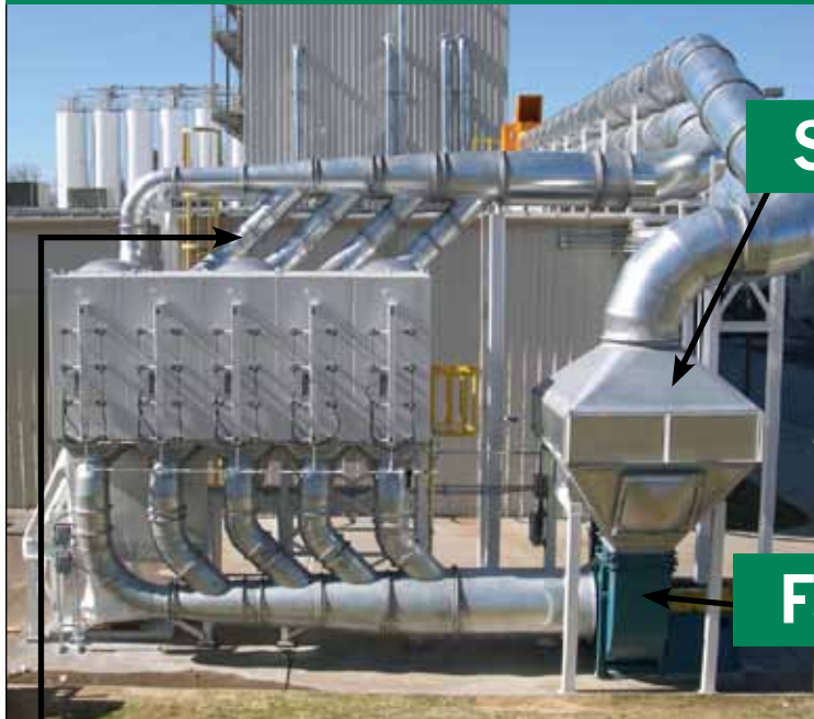
Typical Horizontal Cartridge Filter unit
